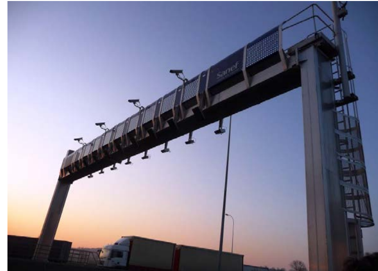
Open Road 'free-flow' tolling gantry – a move away from tolling booths
